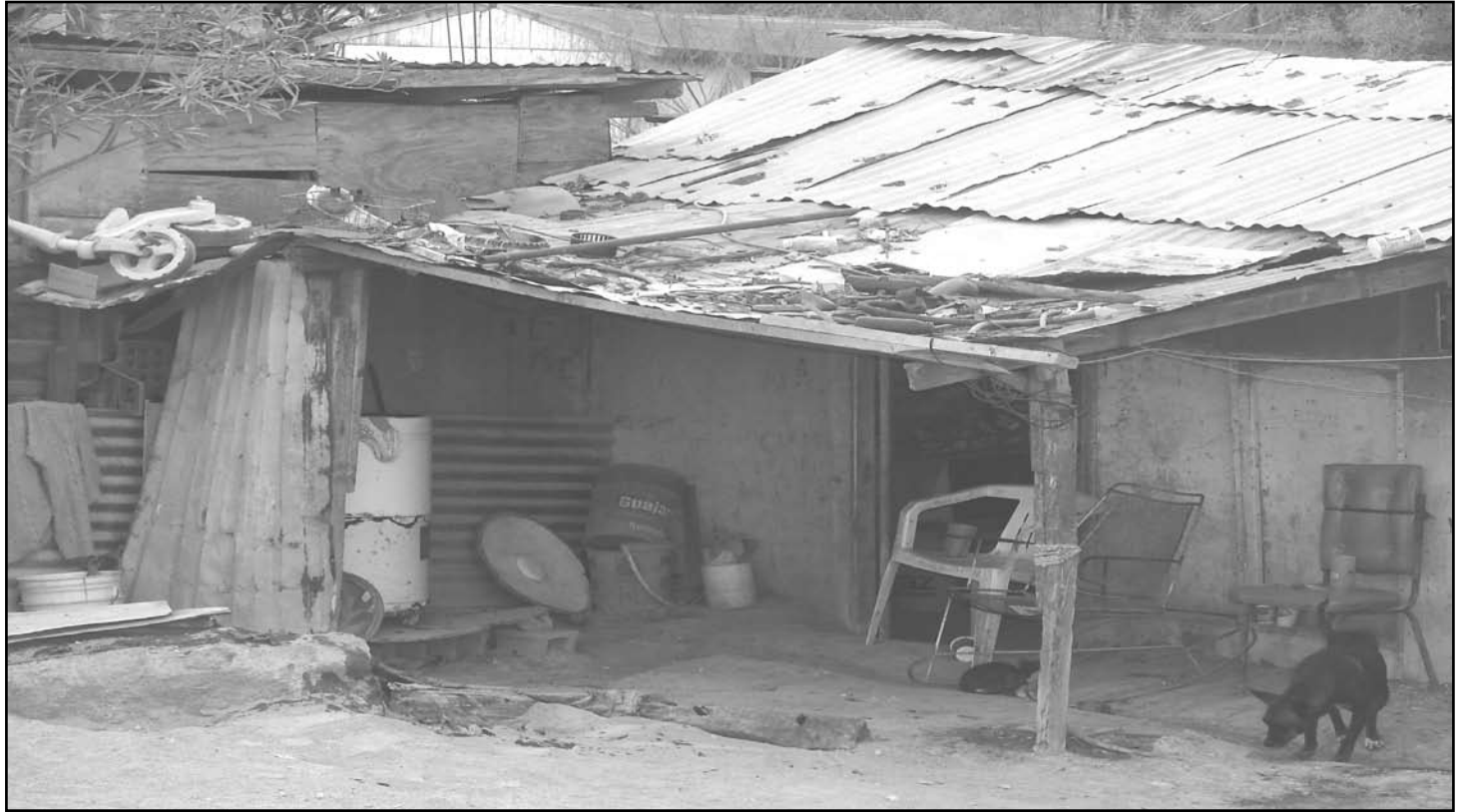
Housing in the colonias or neighborhoods for workers on the US-Mexico border regions is crumbling. Photo by Justin Vitiello.
